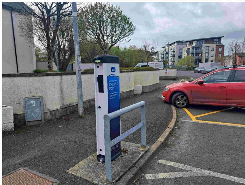
Figure 3.3: EV Charger, Shannon Garda Station
