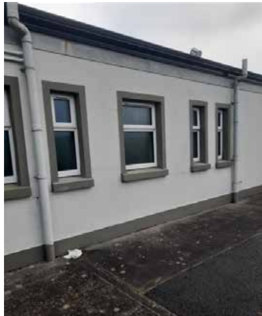
Mike McTigue Community Centre replaced seven old windows with new triple glazed units to improve the energy efficiency of their centre.
