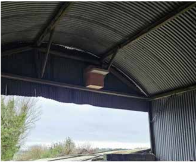
Barn owl nest boxes installed during December 2024 as part of the 'Return to Nature Clare Church Biodiversity Project'.
